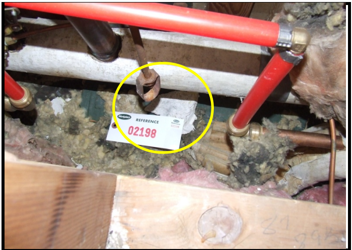
Photo 4 : Asbestos Pipe Fitting Debris 10% Chrysotile Asbestos
