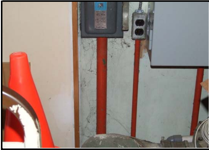
Photo 1 : Red paint on electrical conduit piping HVAC/Boiler Room, South wall
