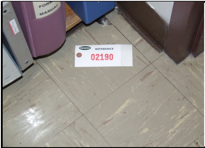
Photo 1 : 9"x9" Gray Floor Tile Both Tile & Mastic Contain 2-3% Chrysotile Asbestos
