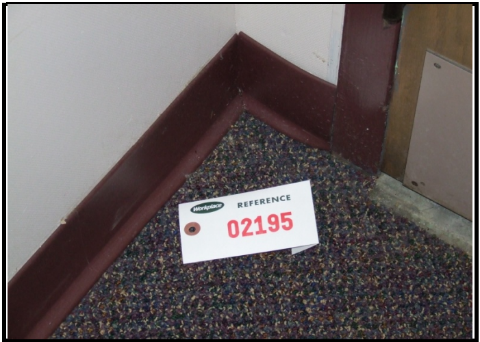
Photo 2 : Carpet Covering Asbestos Black Mastic Contains 3% Chrysotile Asbestos
