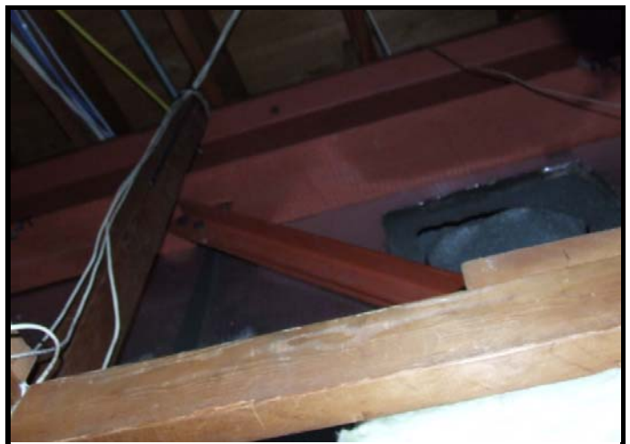
Photo 6 : Burgundy paint on support beams Attic space above the Janitor's Closet
