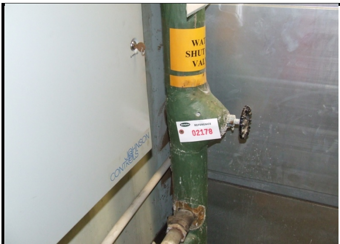
Photo 5 : Non-asbestos Pipe Fitting Insulation HVAC/Boiler Room
